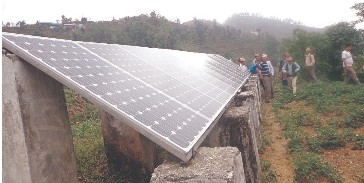
Figure: Solar MUS installed at Jagatbhangjyan 2, Aarupata
